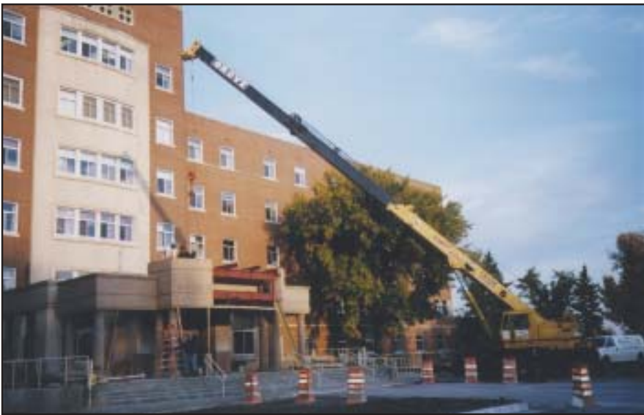
The first concrete block, one of four with the school's name, is lowered into place atop the newly renovated east entrance of the UND medical school. Renovation was funded in part by alumni contributions in honor of former Dean Theodore H. Harwood, M.D.
