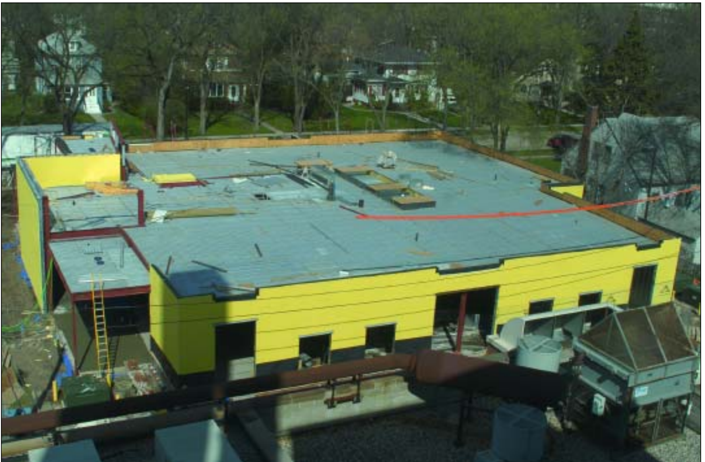
Construction is proceeding on the $3 million Neuroscience Research Facility just west of the UND medical school, on the northeast corner of Fifth Avenue North and Hamline. The one-story building, plus basement, is expected to be completed this fall.
